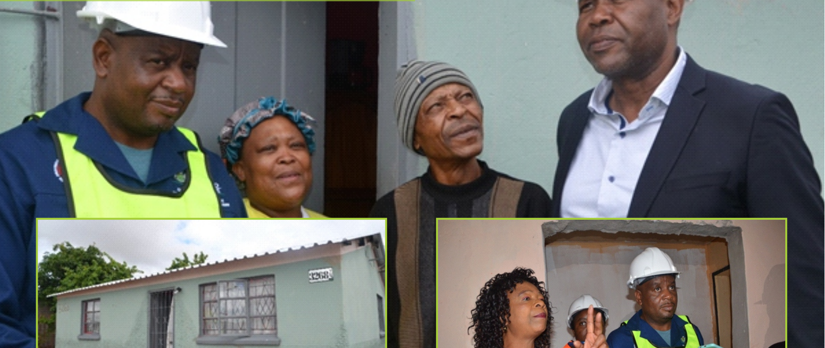
The MEC for CoGHSTA, Mr Basikopo Makamu, residents of Seshego, Ms Lebogang Mashilwane, Mr Andrew Thema and the Executive Mayor of Polokwane Municipality, Cllr John Mpe during a Media Tour to showcase the progress on the removal and replacement of asbestos roofing in Seshego under Polokwane Local Municipality.
